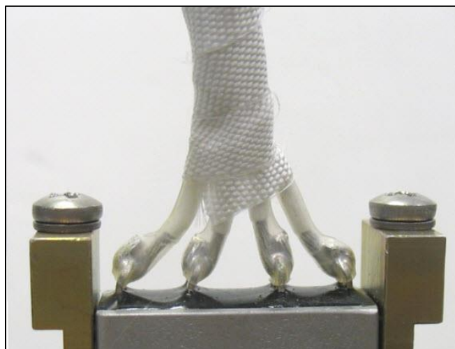
Figure 11: Taped wires exiting switch
